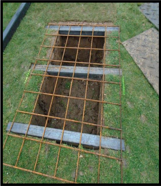
Tubular Supports and Grid
